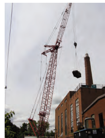
At Smith College, a crane installs components of the new cogeneration system.
